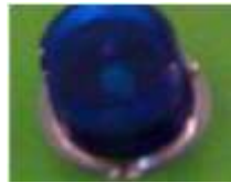
KPE/MCE - Strobe light mounted next to the escape staircase and cross passage doors
