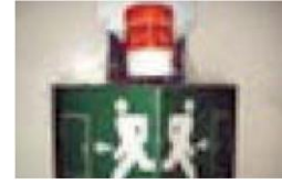
CTE – Strobe light mounted above door
