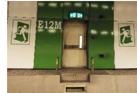
KPE/MCE: In an emergency, look out for white escape staircases and cross passage doors with green walls and identified by flashing bluish-white strobe lights Escape Staircase Cross Passage Door
