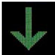
The GREEN Arrow indicates that the lane is open for use
