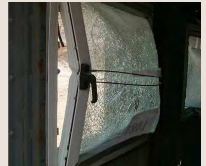
Figure 42: Window after explosion
