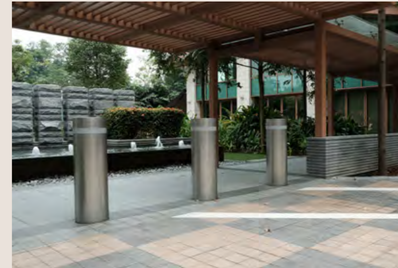
Figure 1: An example of a continuous Vehicle Anti-Ramming Perimeter Line.
