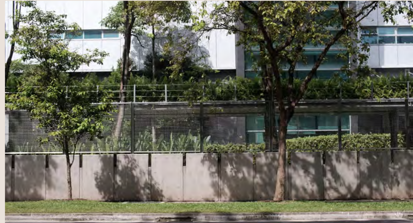
Figure 8: Example of an anti-intrusion perimeter line.
