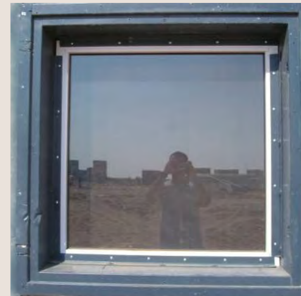
Figure 30: A window protected by mechanically anchored ASF for basic blast level (before explosion)
