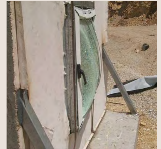
Figure 29: Cable protected window for low blast levels (after explosion)
