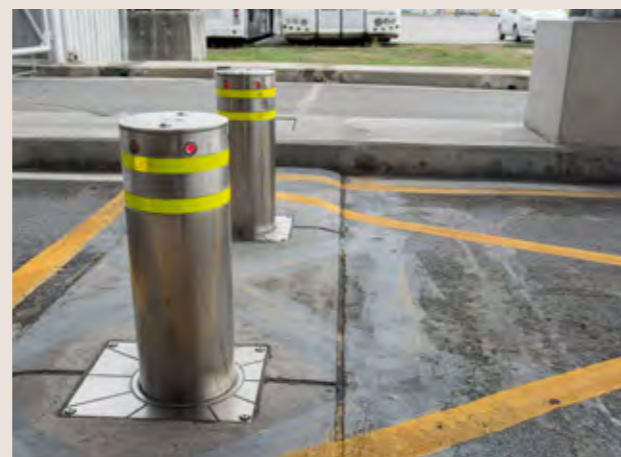
Figure 14: Retractable anti-ramming bollards
